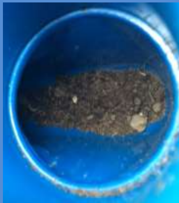
Image of hydrant cup pre clean
