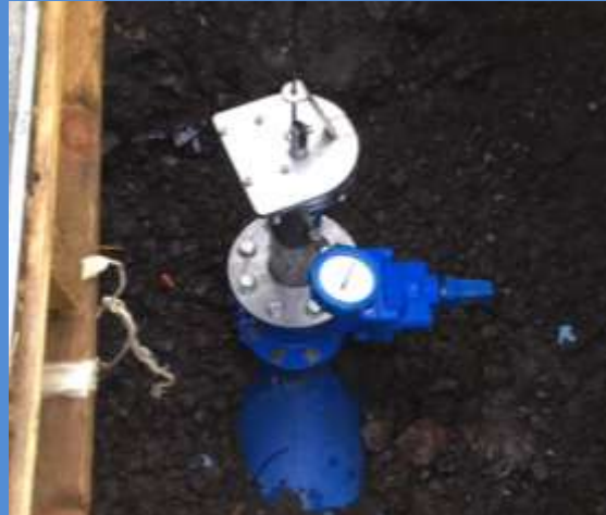
Cable extraction from live water pipe
