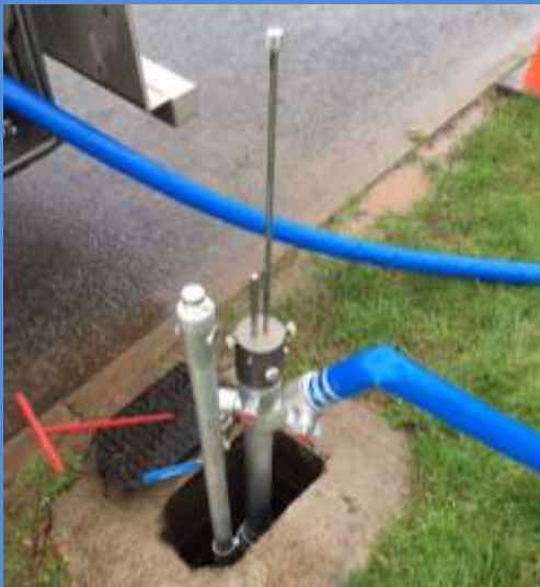
LJK shown on hydrant
